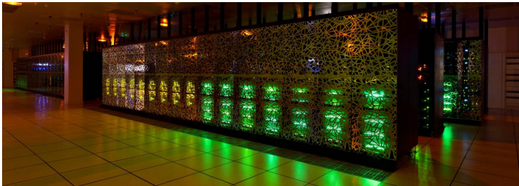
The CURIE supercomputer installed at TGCC
